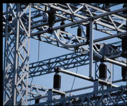
. . . or electrical stations with transformer boxes nearby.
